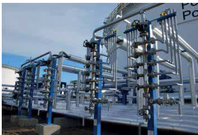
A steam tracing system installed in Poland
